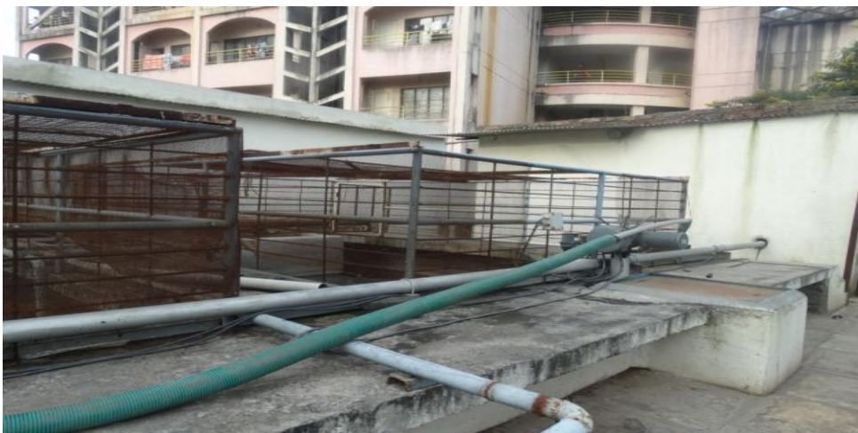
Sewage Treatment plant- I
