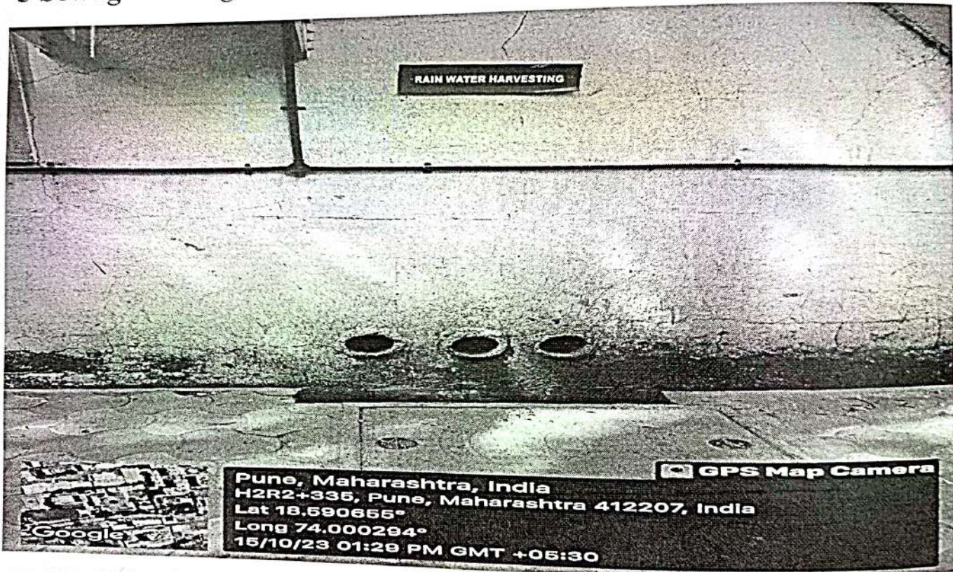
6-Rain Water Harvesting Pipes
