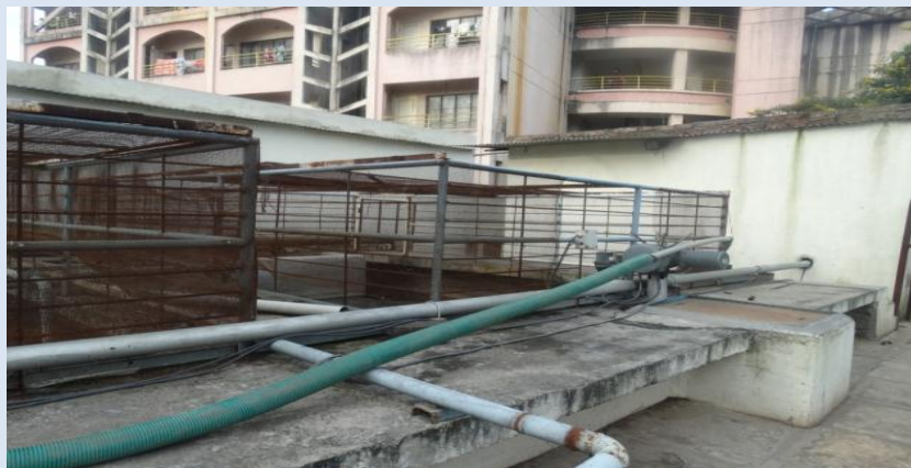
Sewage Treatment Plant- I
